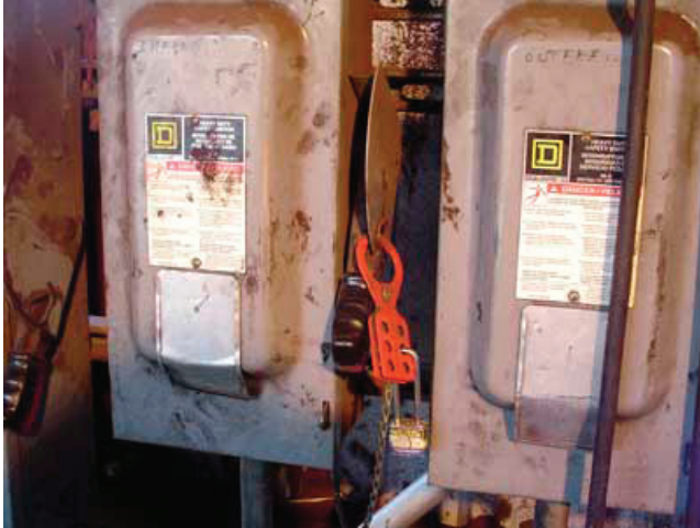
Figure 1. This photo illustrates the south debarker room where locks had been placed on two electrical circuits by the victim [Photo courtesy of SCOSHA].
